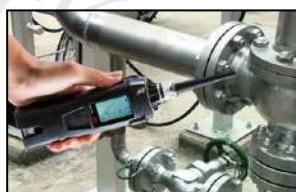
For gas pipe joint
